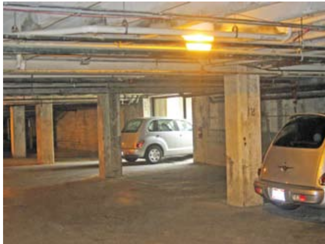
Secure underground parking is available.
